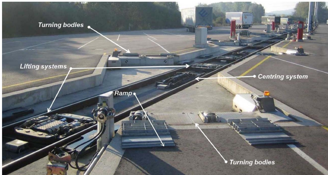
Figure 22. Specialized loading mechanism built into the transshipment track of Modalohr terminal Source: lohr.fr
