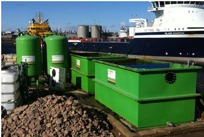
Soilutions_Pump and treat
